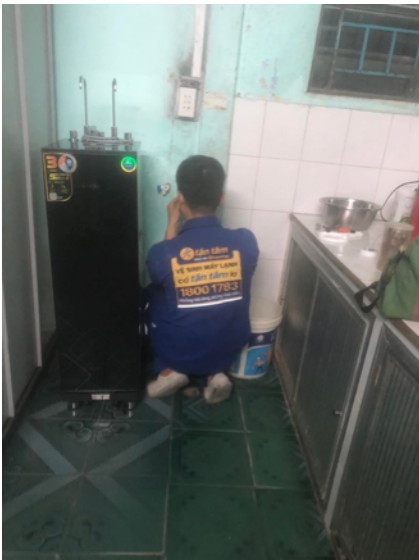
New water purifier, installed in May 2023 – thank you donors!
